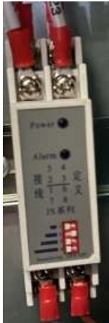
Water leakage detector
