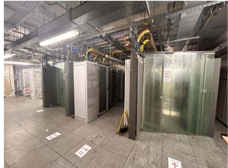
Telecom server room in UK
